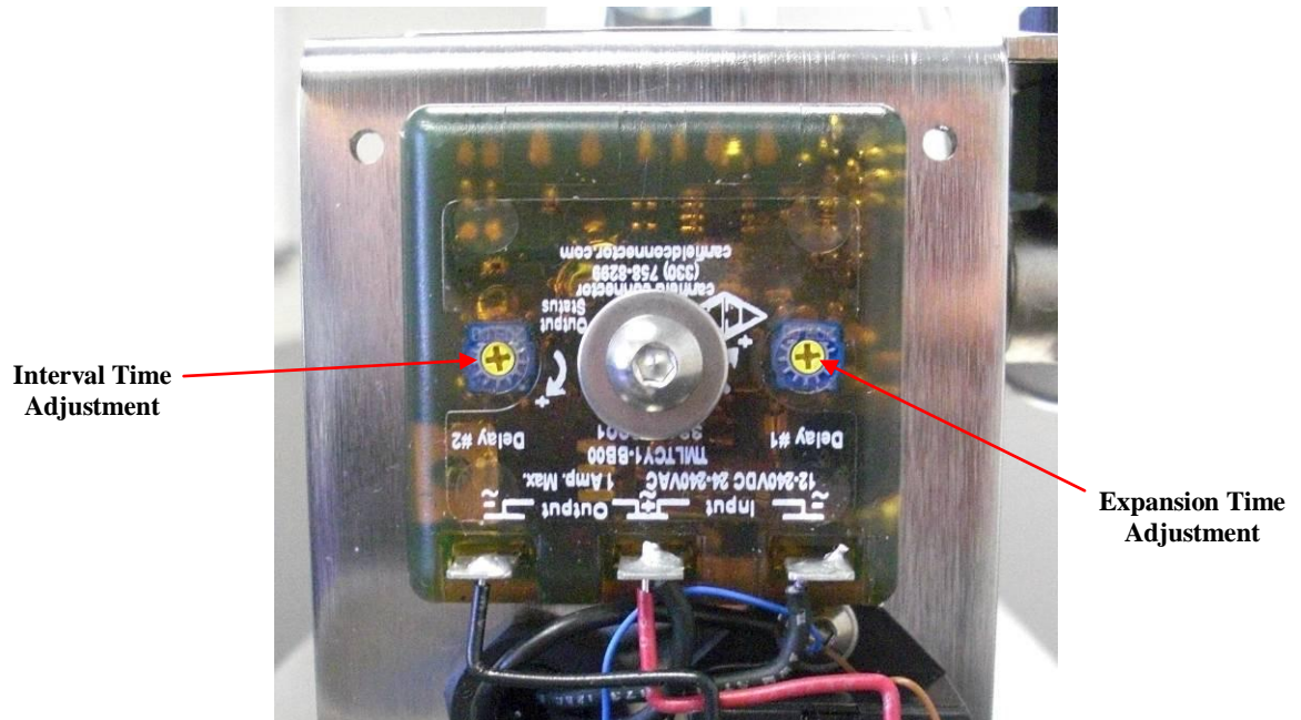
Figure 5: Time Delay Relay and Time Adjustment Pots
